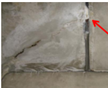
Figure 7: Leaking and leaching concrete
