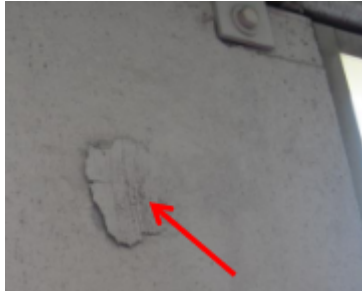
Figure 1: Failing concrete patch
