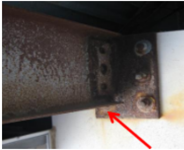
Figure 9: Structural steel rust & scaling
